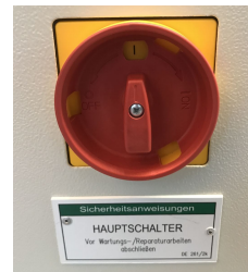
Fig. 15: Example: Main switch for switching the lift on and off
