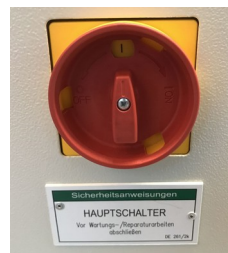
Fig. 20: Example of main switch
