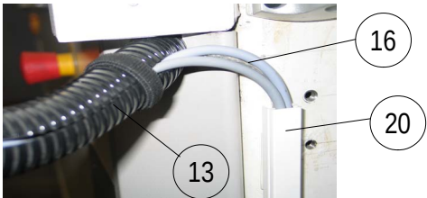
Fig. 15: Customer-side peripheral cables in the cable duct
